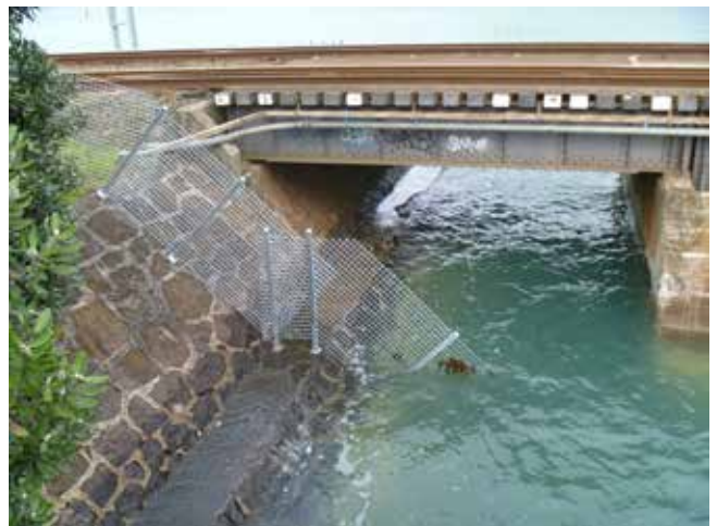
Judges Bay Rail bridge at high tide. The fence goes way underwater.
