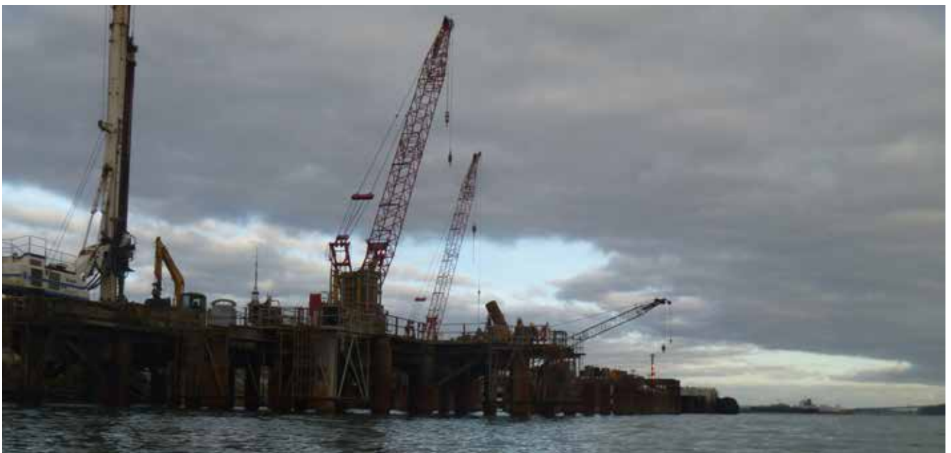
This is the start of a new wharf frontage being built at the end of the Fergusson Container Terminal. We always paddled close in near the old rock sea-wall when paddling past here, the narrowest part of the harbour. With the port expansion encroaching ever further, life will just get that little bit more challenging.
