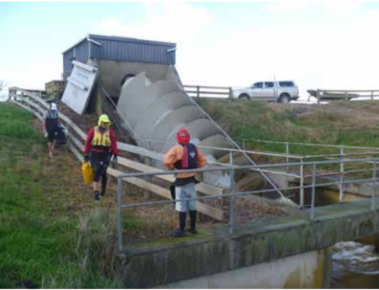
The giant Archimedes screw in action. It lifts water draining out of former swamp-land below Mangatawhiri, into the Maramarua River just beyond the flood bank. That's a spare gearbox for the screw just to the left of the engine-house. The broad flat plate nearby is a spare sluice gate. The Toyota Ute to the right gives some perspective to the scene.
